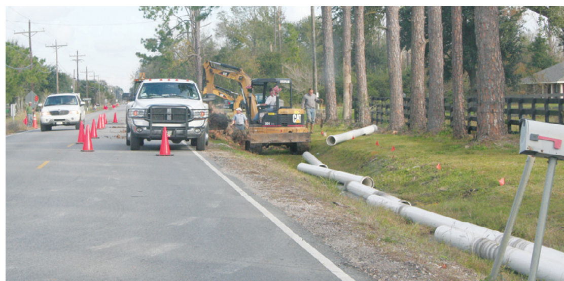
WORK IS PROGRESSING on a major water project in Grand Lake by Waterworks District #11. The 10 inch line upgrade is being funded by a CDBG grant. (Photo by Cyndi Sellers.)
