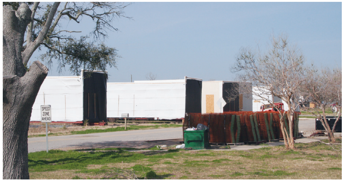
SECTIONS OF the South Cameron Memorial Hospital have arrived in Creole. As soon as weather permits they will be placed on the piers, joined together, and assembled into a complete emergency room with acute care rooms. The hospital hopes to open in March. (Photo by Cyndi Sellers.)
