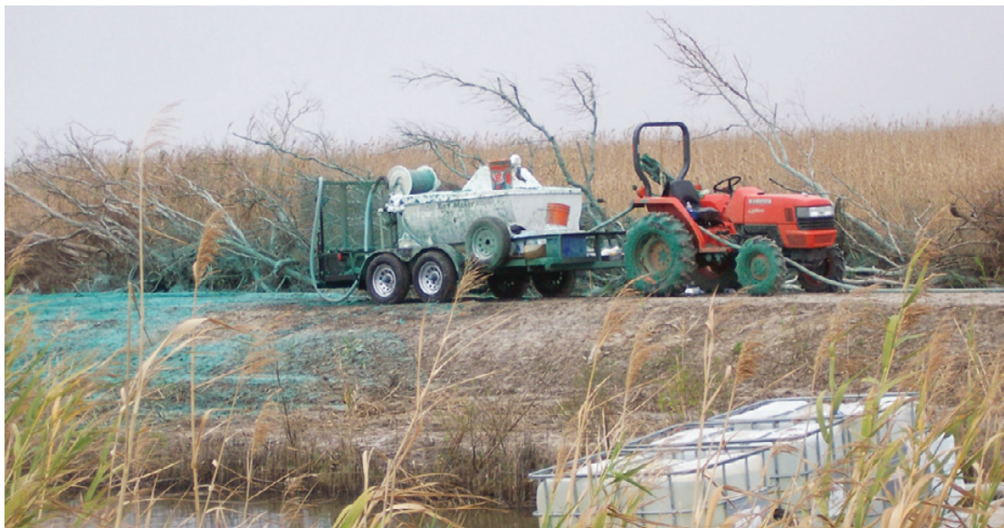
THE LEVEE from the Wetland Walkway northward in the Sabine Refuge has been undergoing renovation. This week grass seed was being spread on the side. (Photo by Cyndi Sellers.)
