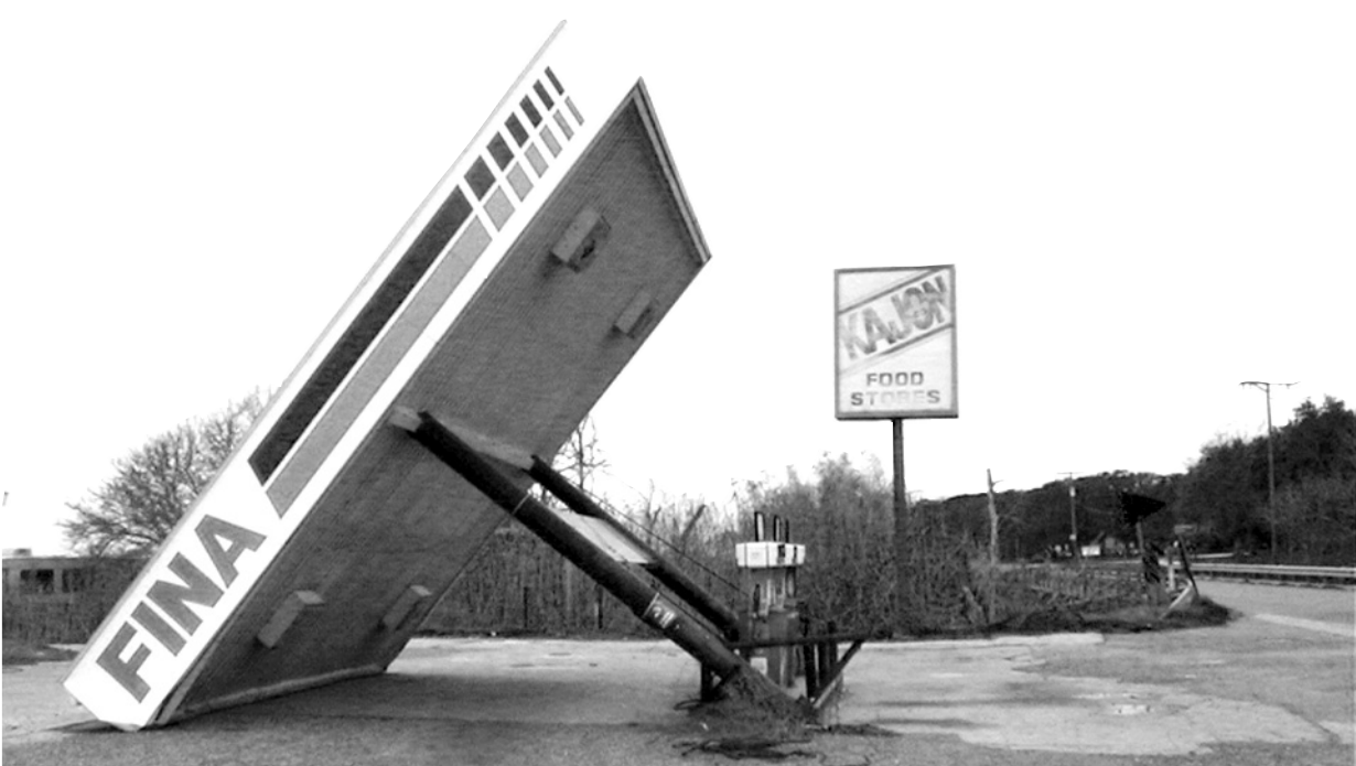
THIS LARGE canopy at the Kajun Food Store at Oak Grove was blown down on Monday, Feb. 5 when a storm front came through. The store has been closed for some months.
