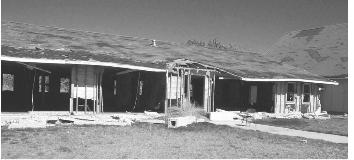
THE CHURCH hall at St. Eugene Catholic Church in Grand Chenier was gutted by the storm. (Photo by Cyndi Sellers.)
