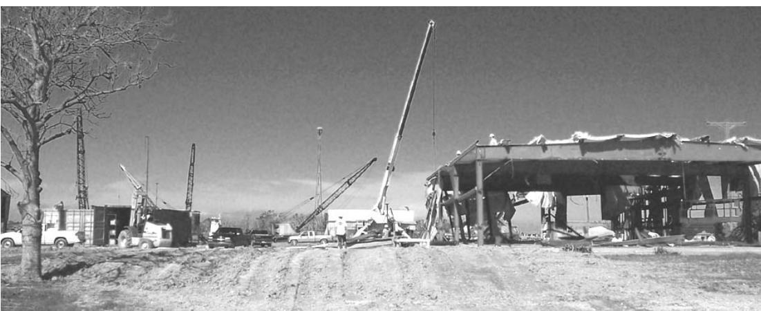
CRAIN BROS. in Grand Chenier is busy repairing its facility. (Photo by Cyndi Sellers.)
