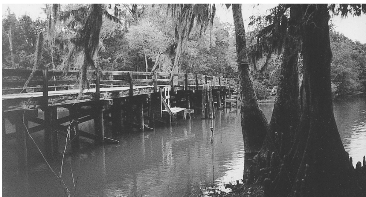
THE LORRAIN BRIDGE over Lacassine Bayou, although located in Calcasieu Parish, has had close connection to Cameron Parish over the years. Back in the '40s it was used to cross cattle moving between Sweetlake and Welsh areas. Efforts are being made to restore the old bridge.
