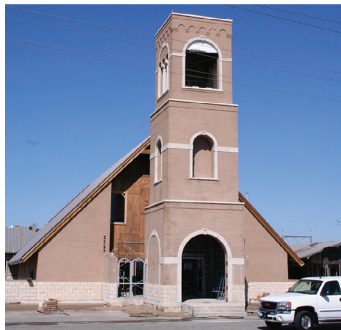
SACRED HEART Catholic Church in Creole, which was almost completely destroyed in Hurricane Rita in 2005, is now being restored. A new bell tower is now taking shape in front of the building. (Photo by Cyndi Sellers.)
