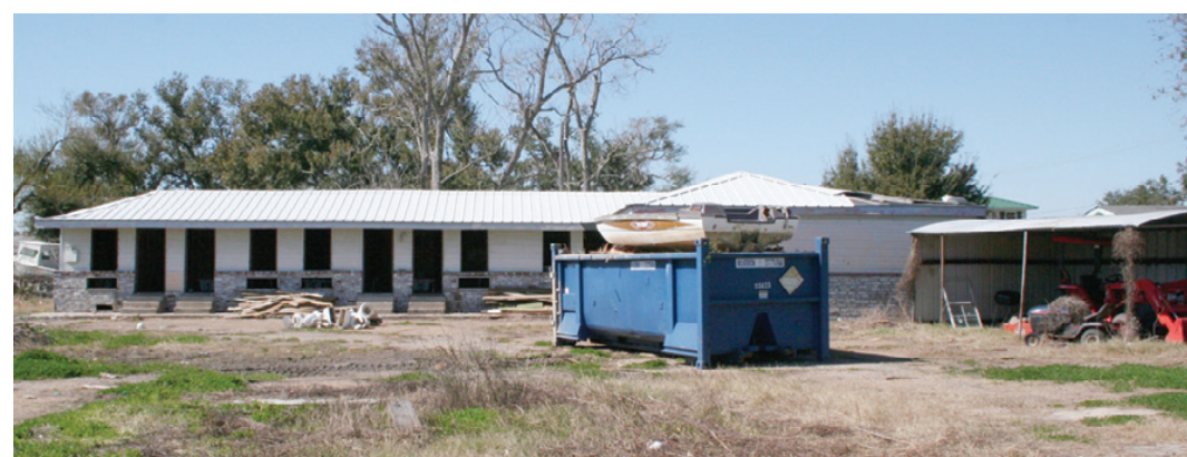
INTERIOR DEMOLITION and site clean-up is under way at the former Cameron Motel #2, in Cameron, which is being remodeled into apartments by new owners Stephen and Margie Vincent. With FEMA about to close its trailer parks, more rental properties will be welcome in Cameron. (Photo by Cyndi Sellers.)
