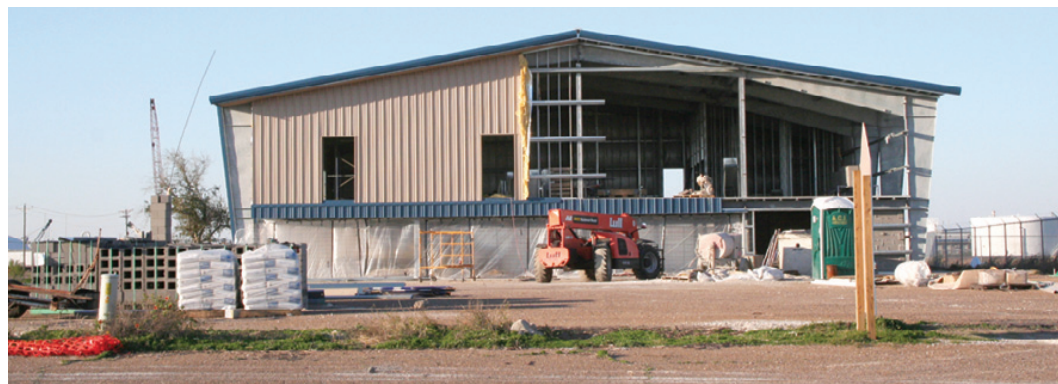
THE NEW and improved Johnson Bayou Community Center is taking shape. (Photo by Paul Sellers)
