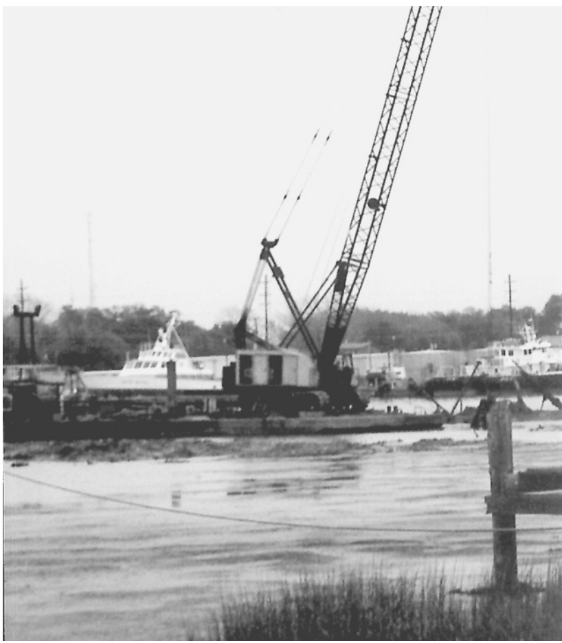
A DRAGLINE IS shown cleaning up the derelict boats that have been deserted along a stretch of the Calcasieu River along the Monkey Island waterfront. (Photo by Geneva Griffith.)
