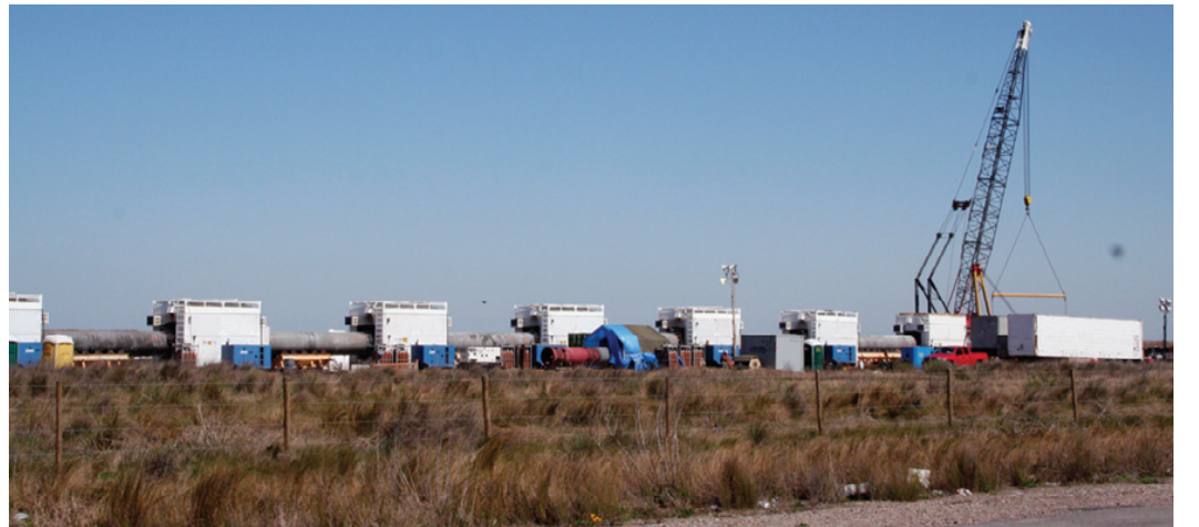
PIPELINE WORK along Hwy 82 near Holly Beach. The 42 inch pipeline is being built for the Sabine Pass Liquefied Natural Gas facility in Johnson Bayou. (Photo by Cyndi Sellers.)
