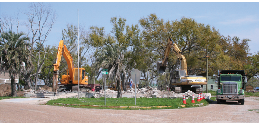
CONCRETE DEMOLITION has begun at the site of the new Police Jury building, to be built on the former site in Cameron. (Photo by Cyndi Sellers.)
