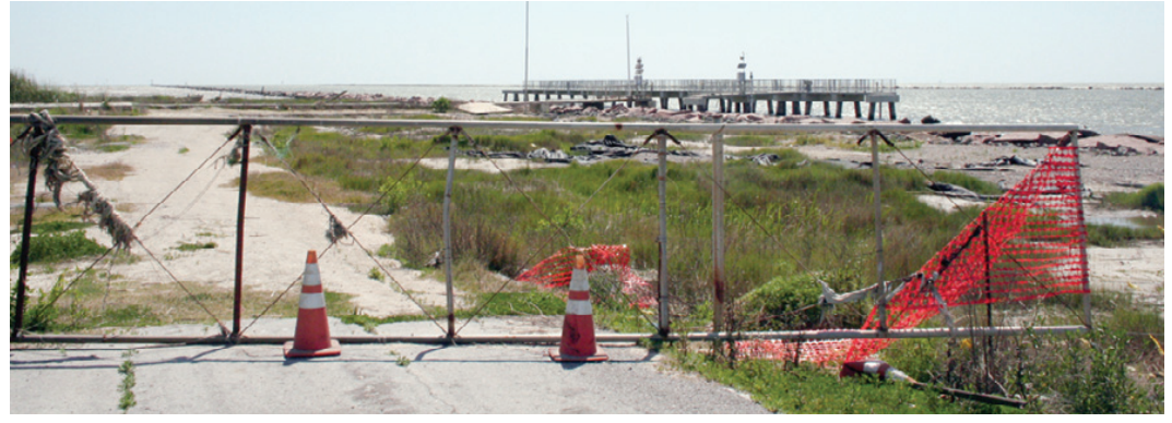
THE JETTY PIER has been closed since Hurricane Rita. Some parts of the repair project are almost ready to go out for bid. (Photo by Cyndi Sellers.)
