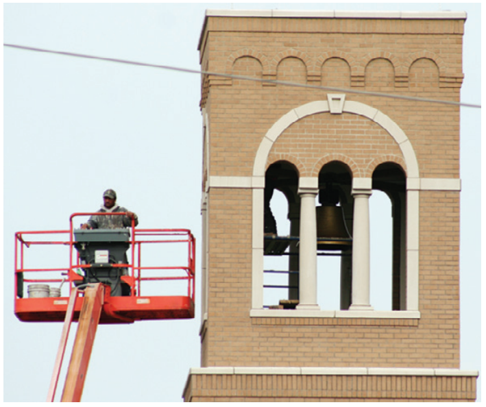
WORKERS INSTALLED the bell in the new bell tower at Sacred Heart Catholic Church in Creole this week. The tower is a new feature for the church, being added along with hurricane renovation.
