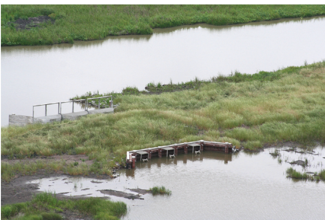
A CWPBRA PROJECT designed to allow fresh water to flow from White Lake in Vermilion Parish, under Hwy. 82 and into the Rockefeller Wildlife Refuge was dedicated Friday. This water control structure will allow fresh water to flow south when there is positive pressure on the north side, countering the effects of salt water intrusion. (Photo by Cyndi Sellers.)
