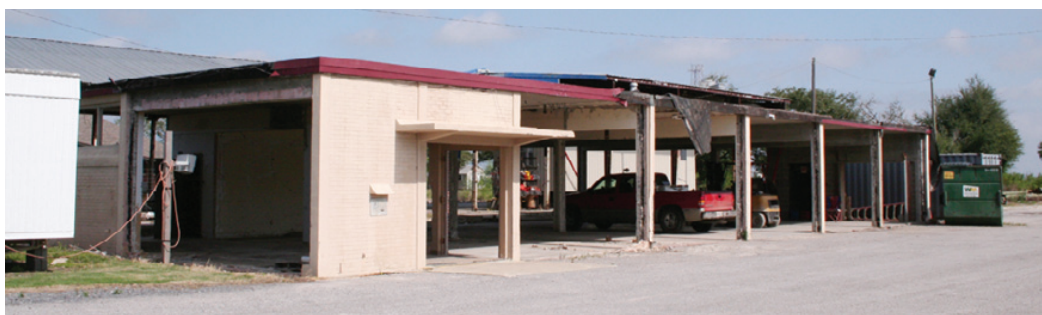
THE JEFF DAVIS Electric Co-op office building and complex are to be rebuilt in Cameron on the original site. It was a total loss following Hurricane Rita in 2005. (Photo by Cyndi Sellers.)
