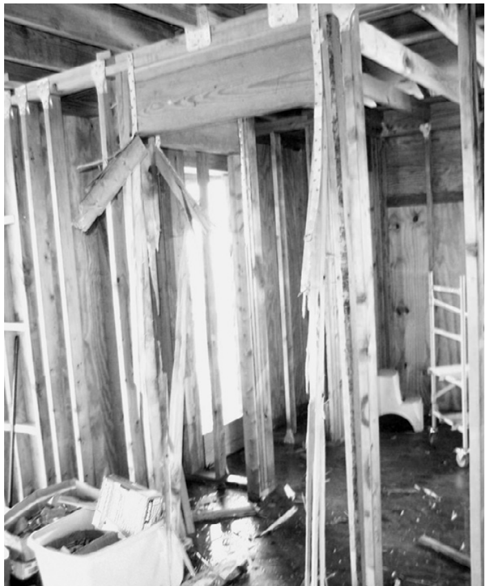
SPLINTERED WOOD and bent metal are the result of a lightning strike on Spencer Owens' house in Holly Beach Thursday morning, May 15. The home is under construction, but damage running from the roof to the ground will have to be repaired before work can continue. (Photo by Cyndi Sellers.)
