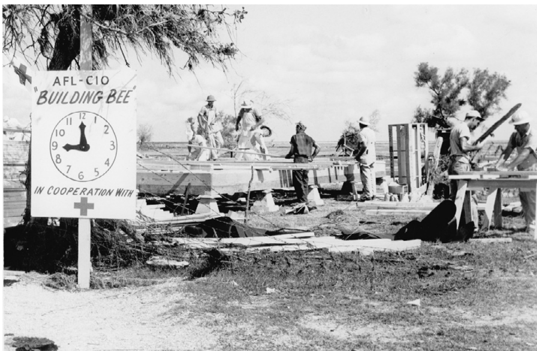
FOLLOWING HURRICANE Audrey help for Cameron Parish residents who lost their homes poured in from all over the country. This photo showed AFL-CIO volunteers partnering with the Red Cross to build homes for the storm victims.
