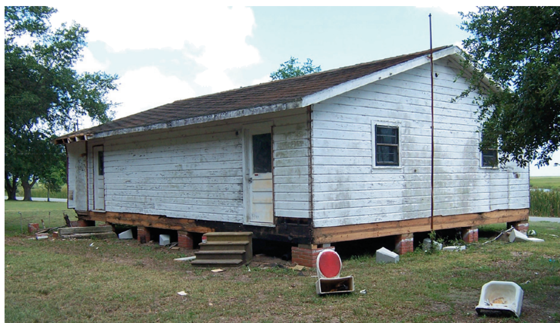
WORK HAS BEGUN on the Grand Chenier Branch Library. The contractor has raised the building to meet FEMA guidelines and removed the small back porch restroom. The next step will be to remove the old roof material and add a meeting room and new back porch onto the rear of the building. (Photo by Cyndi Sellers.)
