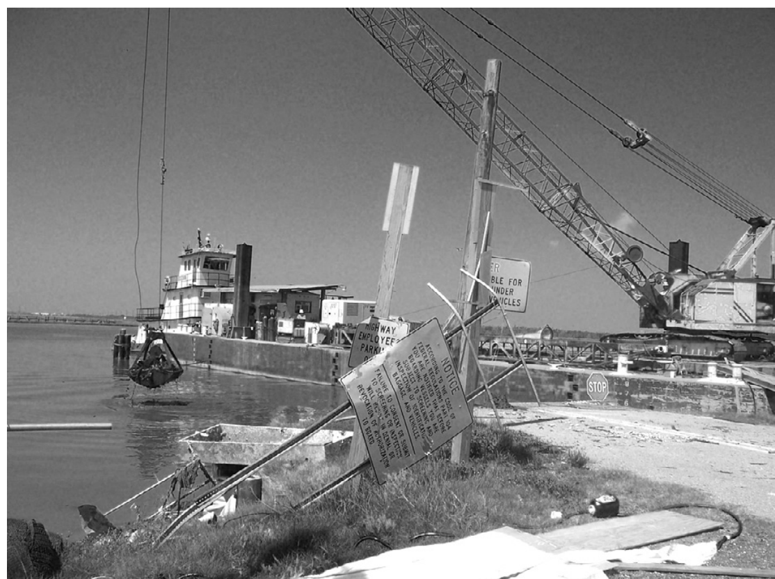
WORK HAS BEGUN on cleaning out the Monkey Island ferry landings. Demolition and cleanup of storm debris is set to begin on the island this week. (Photo by Cyndi Sellers.)
