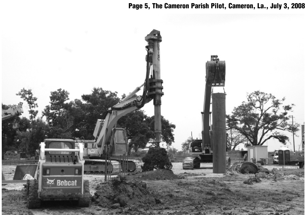
A GIANT AUGER drills holes Monday for pilings to be poured at the site of the new East Annex on Couthouse Square in Cameron. The large pipe on the right is the form for the reinforced concrete, below ground pilings that will support the structure. (Photo by Cyndi Sellers.)
