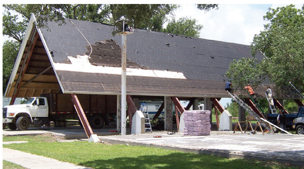
THE CONTRACTOR began work this week on rebuilding the Wakefield Methodist Church in Cameron. Plans are to rebuild only the section under the surviving roof, adding classrooms and other amenities. (Photo by Cyndi Sellers.)
