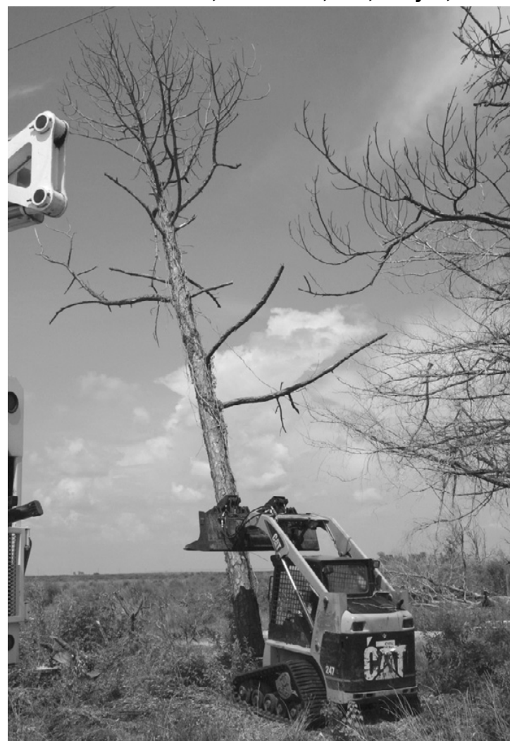
SALT-WATER-KILLED trees are being removed from private property in Cameron by a private contractor hired by the Police Jury. The cost of the tree removal is being covered by FEMA. (Photo by Cyndi Sellers.)
