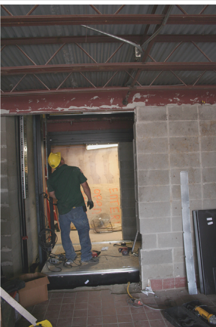
WORKMEN ARE shown installing a new elevator in the Cameron courthouse. The old elevator was badly damaged by Hurricane Rita 20 months ago. The elevator is primarily used by persons ascending to the courtroom on the courthouse's third floor. It is the only elevator in the parish. (Photo by Cyndi Sellers.)
