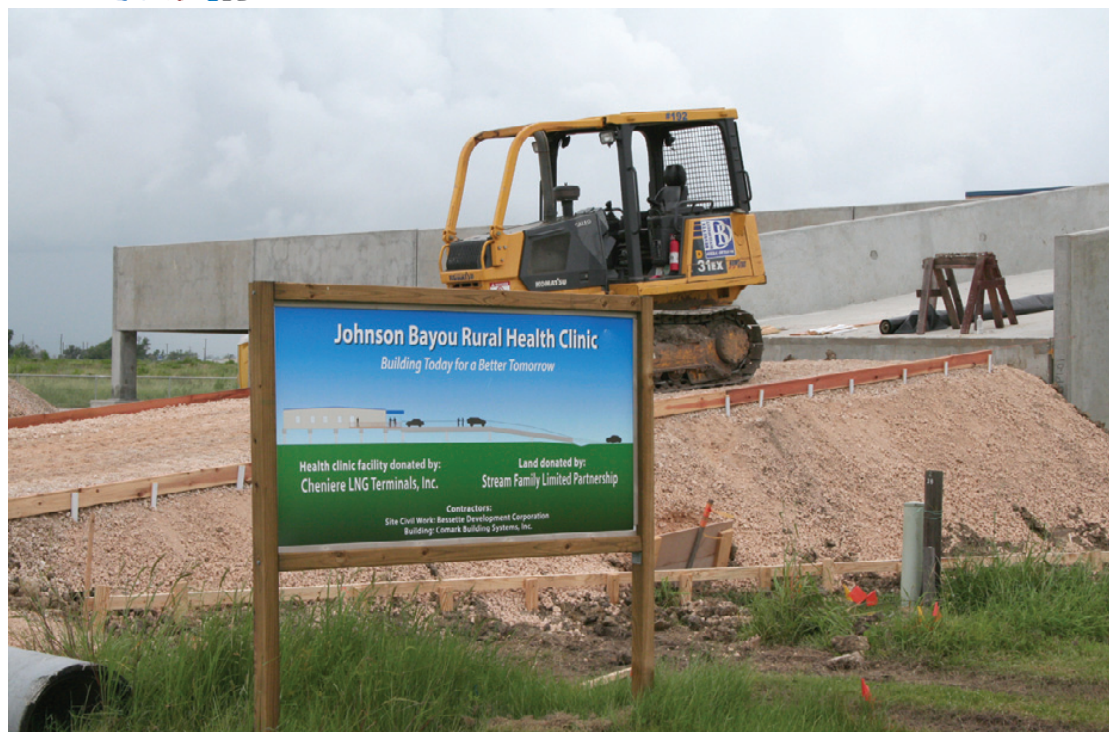
WORK IS progressing on the medical clinic being built in Johnson Bayou by Cheniere Energy. The entire parking lot will be elevated for easy access to the clinic. (Photo by Cyndi Sellers.)
