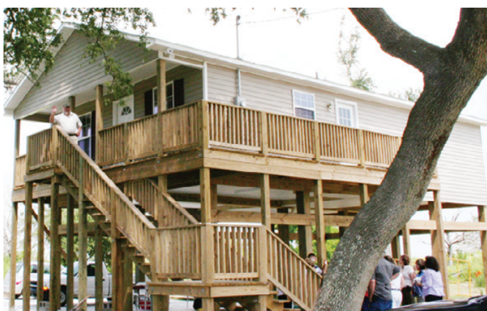
CECIL AND LESLIE Clark are the owners of this new home, built by SWLA Habitat for Humanity and the Louisiana Catholic Daughters. It was the first house Habitat has built on pilings, and presented special challenges to the builders. The house stands on the site of the home of Clark's father, the late Dr. Cecil Clark, well remembered for his heroism during Hurricane Audrey. (Photo by Cyndi Sellers.)
