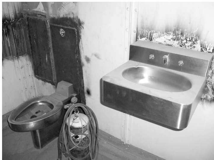
PLUMBING REPAIRS are nearly complete at the Cameron Parish jail, and final reconstruction has begun. New pipes and stainless steel fixtures have been installed and the entire jail has been prepared for repainting. (Photo by Cyndi Sellers.)
