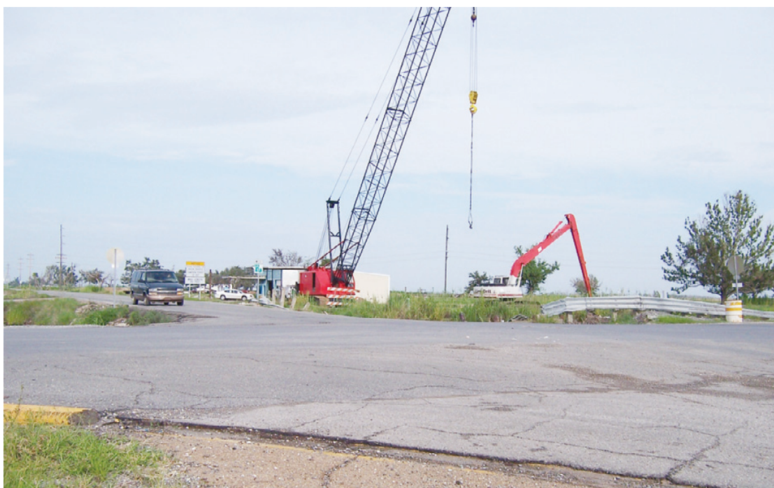
WORK ON THE bridge at Oak Grove has begun. (Photo by Cyndi Sellers.)
