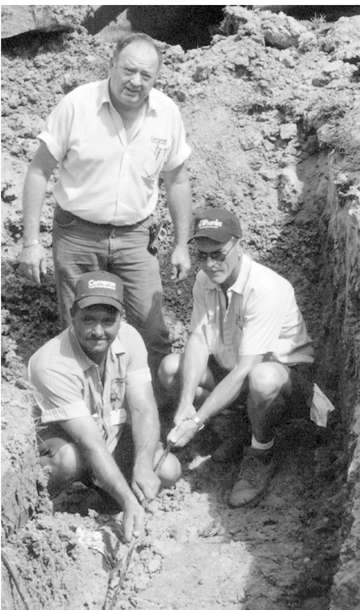
CAMERON COMMUNICATIONS' technicians Jerry Waite, Steve Poole and Tony Frederick make the first splice to connect Cameron Communications' FTTH in Grand Lake to their existing fiber optic ring, supplying residences with PowerHouse voice, video and Internet connectivity.
