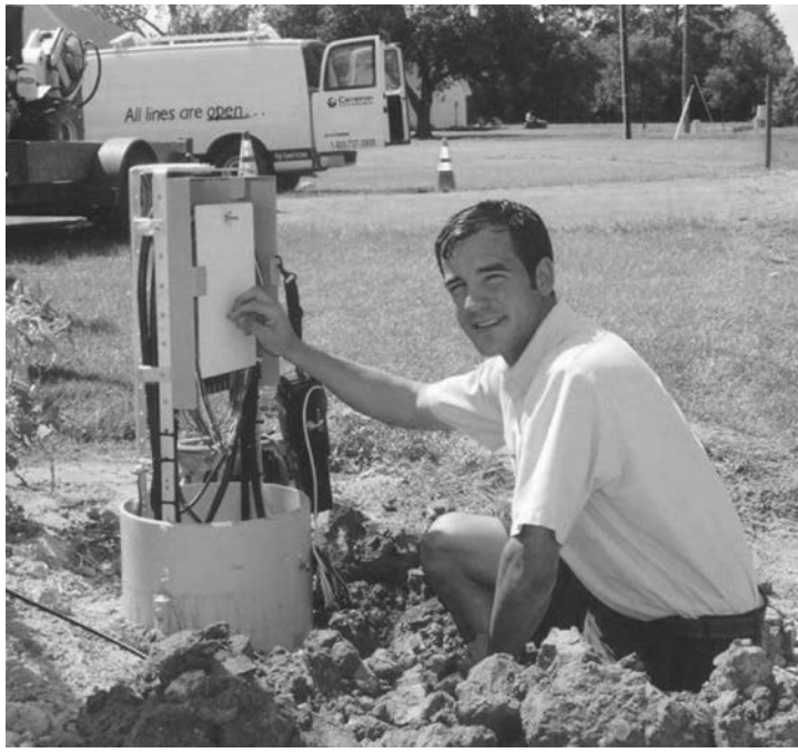
Cameron Communications' continues work on their 3-phase FTTH project in Grand Lake that began in July of 2004 and should be completed by fall of 2005.
