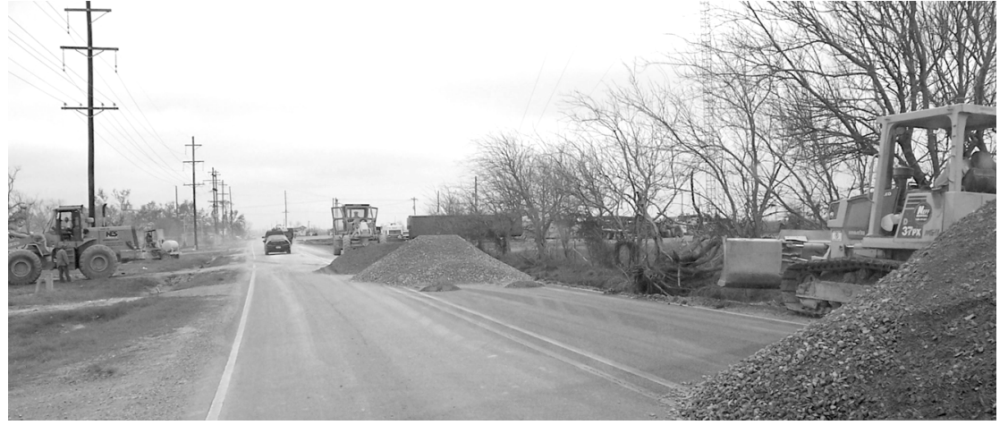
SHOULDER REPAIR IS nearly complete along Hwy. 27 between Creole and Cameron. Repairs have allowed the School Board to resume a bus route from Cameron to Grand Lake. The bus leaves the Court House at 6:50 am. (Photo by Cyndi Sellers.)
