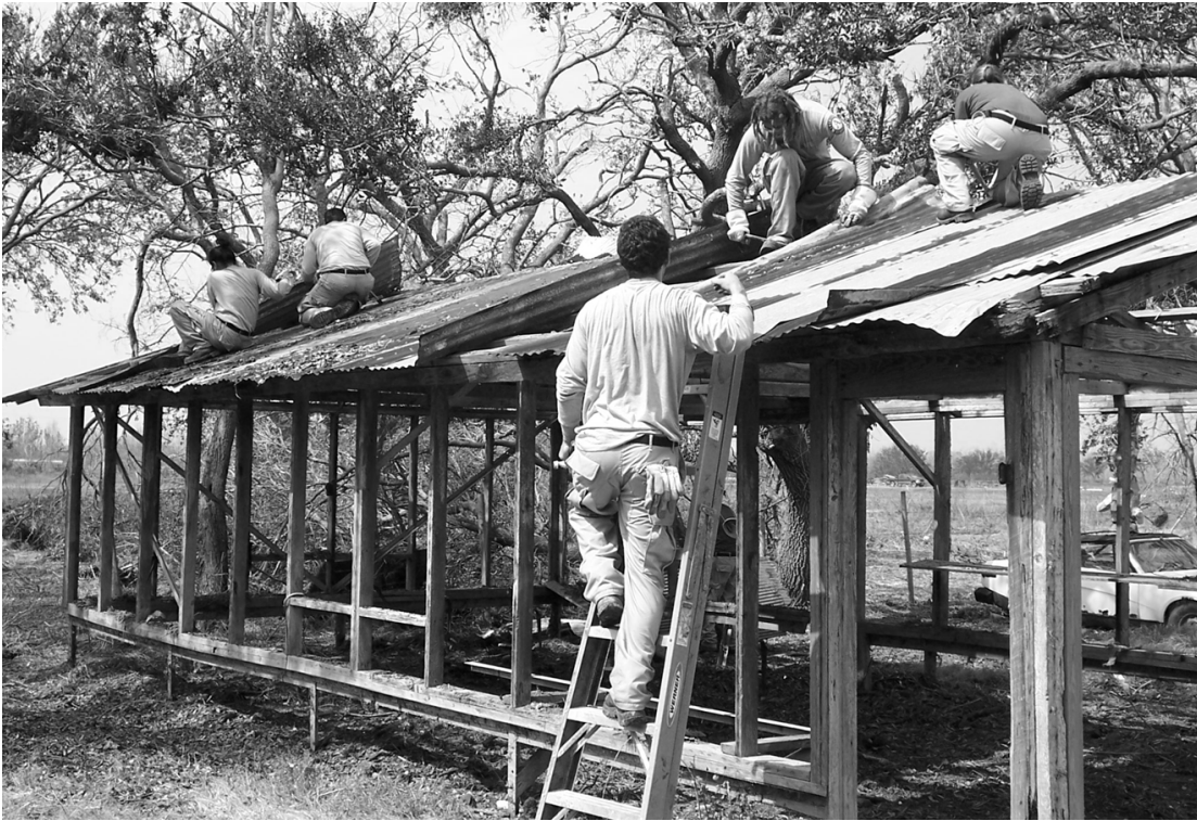
AMERICORPS TEAMS were working in Hackberry on Monday helping residents clean up storm debris. This team was at the home of Gerald and Joe Ann LaBove where they took down a shed, cleaned out a barn, and picked up debris from a fence line. Joe Ann said she didn't know how it would have gotten done without the team's help, since Gerald has health problems and the debris was too heavy for her and her children. For help with clean-up of storm damage, call Julie Burleigh at the Cameron EOC, 775-7770, or Dinah Landry at the Council on Aging, 905-5000. (Photo by Cyndi Sellers.)
