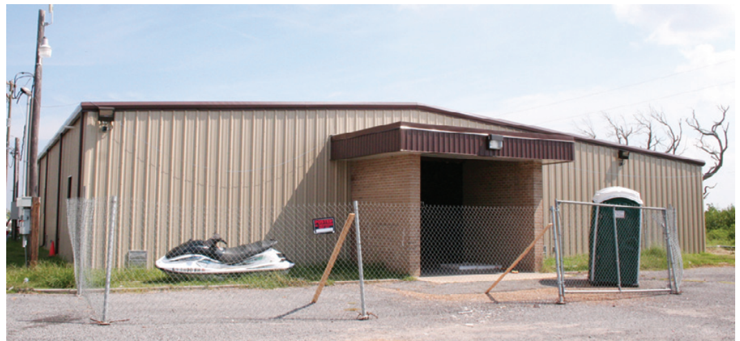
THE CAMERON Multipurpose Building is closer to completion, but the contractor has asked for an 84 day extension due to unforeseen repairs and weather stoppages. The request was one of several plan changes causing concern at Monday's Police Jury meeting. (Photo by Cyndi Sellers.)
