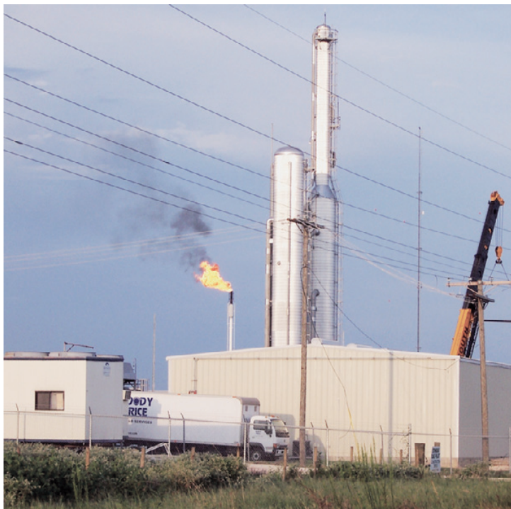
THE FLARE AT the Stingray Pipeline in Johnsons Bayou highlights operations at the the restored facility. (Photo by Cyndi Sellers.)
