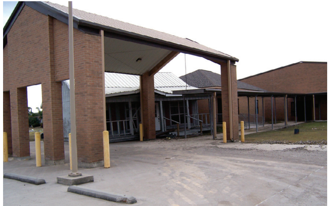
CECIL SANNER'S office was wedged between buildings at St. Peter the Apostle Catholic Church in Hackberry by Hurricane Ike. (Photo by Paul Sellers.)
