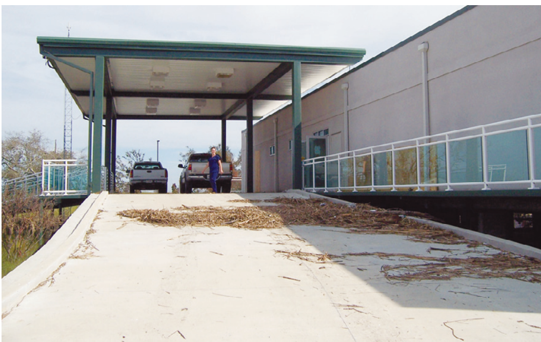
THE DEBRIS on the entrance ramp of South Cameron Memorial Hospital shows the level reached by the flood waters of Hurricane Ike. Staff is already checking out the readiness of the hospital. Photo by Cyndi Sellers.)
