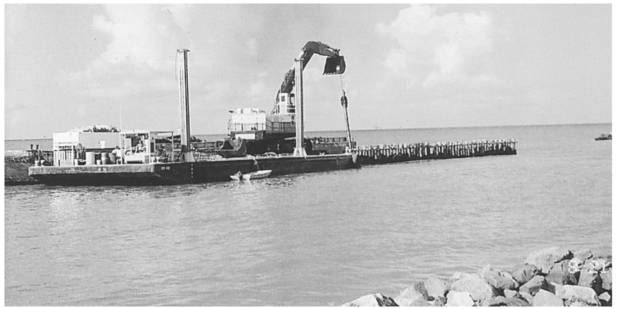
BERTUCCI BROTHERS used barges and trackhoes to remove 6 experimental breakwaters of pilings, rocks, and tires installed in 1984 at Peveto Beach so that Weeks Marine can pump in sand for the Holly Beach-Peveto Beach-Constance Beach project. Pumping of sand has begun.
