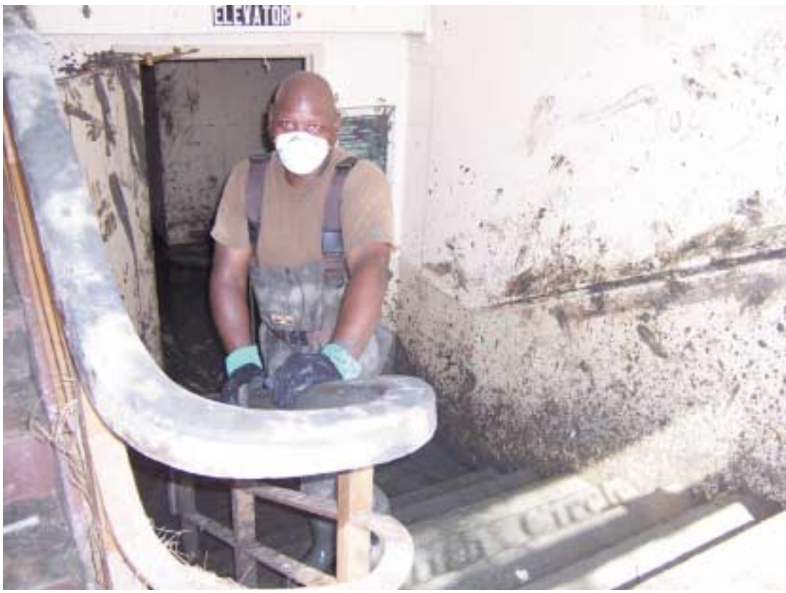
AN ALABAMA National Guard member is shown helping with the cleanup at the Cameron Parish Courthouse. This shows the basement level of the courthouse, which was completely flooded. The building's main and top floors were not flooded. The courthouse was one of the few buildings in Cameron to survive more or less intact. (Photo by Cyndi Sellers.)
