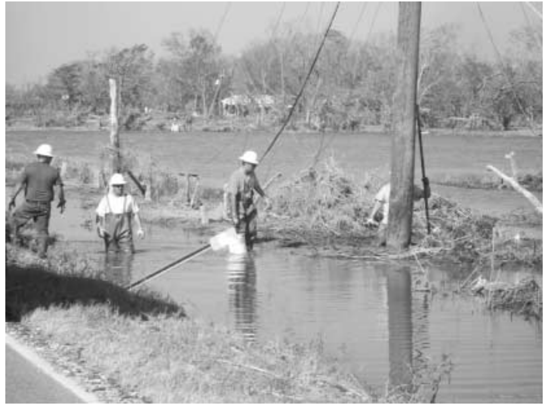
UTILITY WORKERS from 17 states are in the Cameron Parish area restoring electrical service. The above photo taken in Cameron shows the difficulties under which they are working. (Photo by Cyndi Sellers.)
