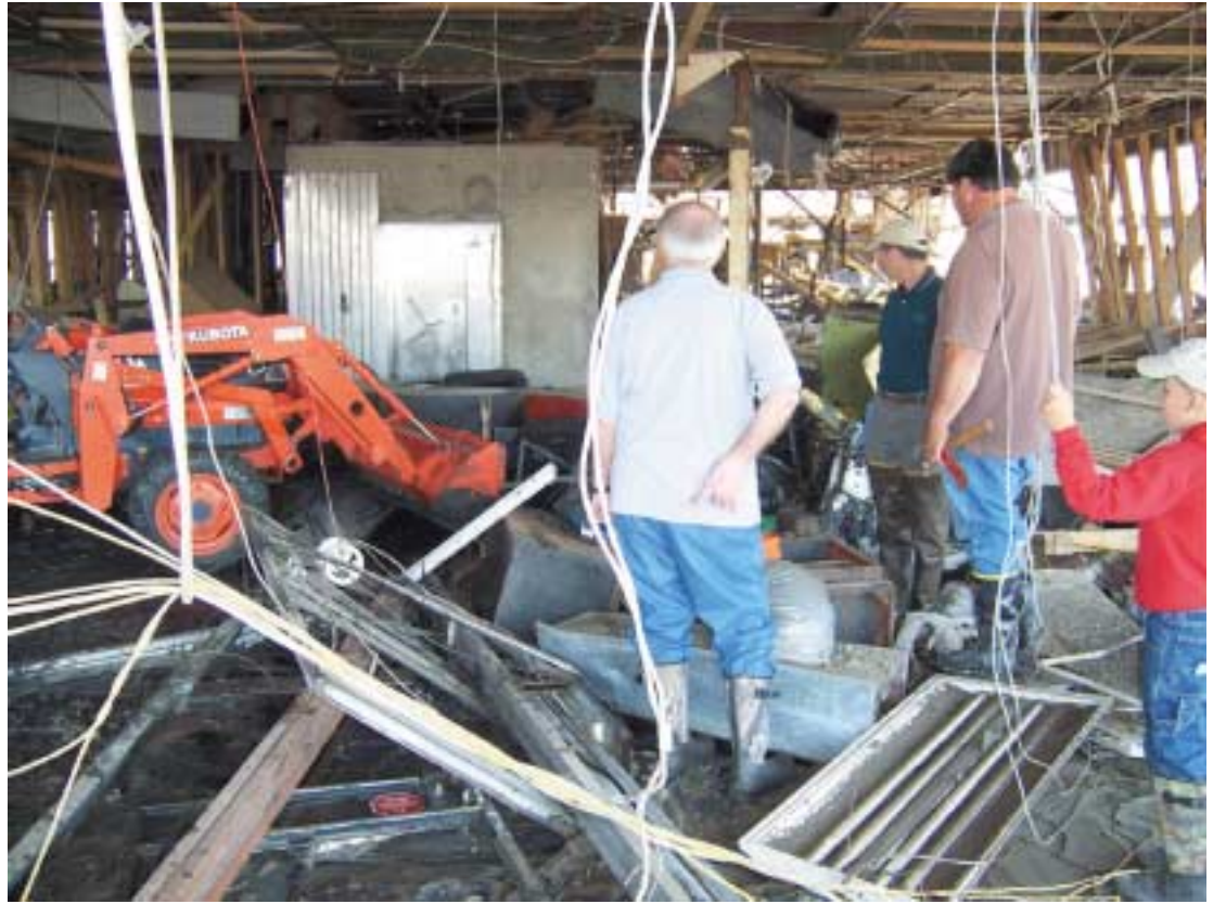
THE CAMERON STATE Bank's Cameron office was completely gutted by Hurricane Rita, as were branches in Creole and Grand Chenier. Here bank officials try to access the vault in Cameron. (Photo by Cyndi Sellers.)
