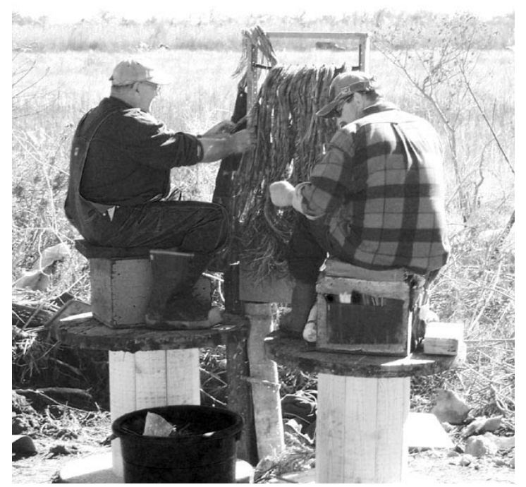
THESE PHONE technicians from Wisconsin represent many such teams now working in lower Cameron Parish to restore the connections damaged by salt water. There are 900 splices to be made in each box. (Photo by Cyndi Sellers)
