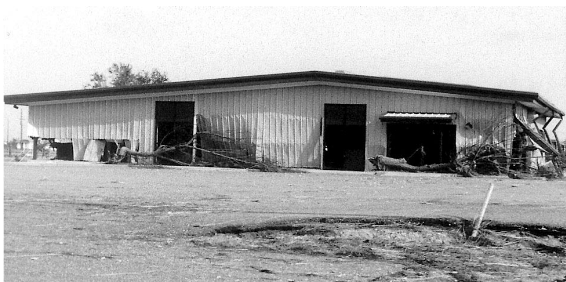
THE JOHNSON BAYOU Community Center was severely damaged by Hurricane Rita although the building remained standing. (Photo by Rhonda Morrison.)
