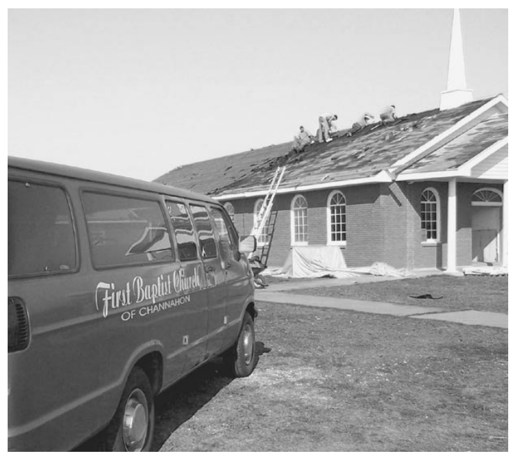
VOLUNTEERS FROM Channahon, Illinois, near Chicago, are helping repair the roof of First Baptist Church of Johnson Bayou. Team leader Kenton Ayers has 40 - 50 volunteers on site. Istrouma Baptist Church of Baton Rouge is supporting the team's effort. Pastor Les Fogleman says two Sunday services have been held so far in the building, which had three feet of flood water and marsh debris. Firemen from Roanoke, Virg., removed the carpeting and Pastor's Council Resource cleared debris. (Photo by Cyndi Sellers.)
