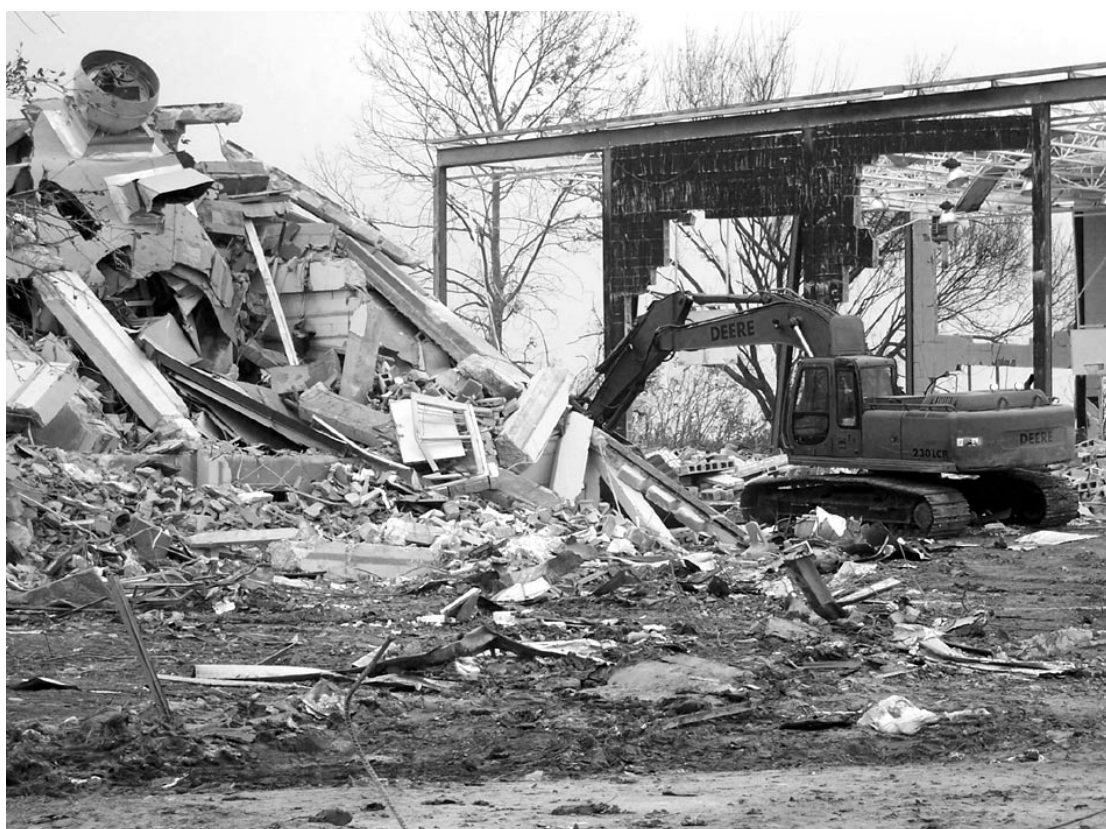
DEMOLITION OF the Cameron Elementary School has begun. The Louisiana National Guard is conducting the demolition. (Photo by Cyndi Sellers.)
