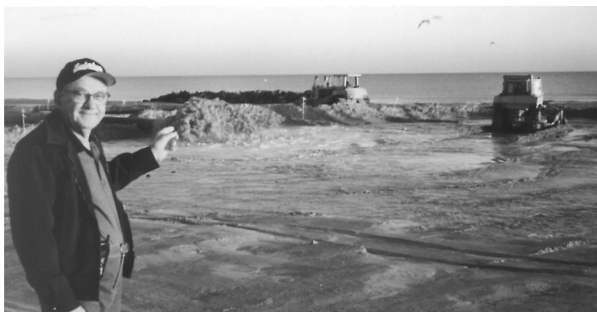
CONSTANCE BEACH resident Rodney Guilbeaux here points out the work being done on the beach nourishment project being carried out by the state between Constance and Holly Beaches. Weeks Marine, the general contractor, has completed the work on the east side of the project and is now heading west. Sand is being pumped from offshore to restore an area of the beach that has been badly eroded in the past.
