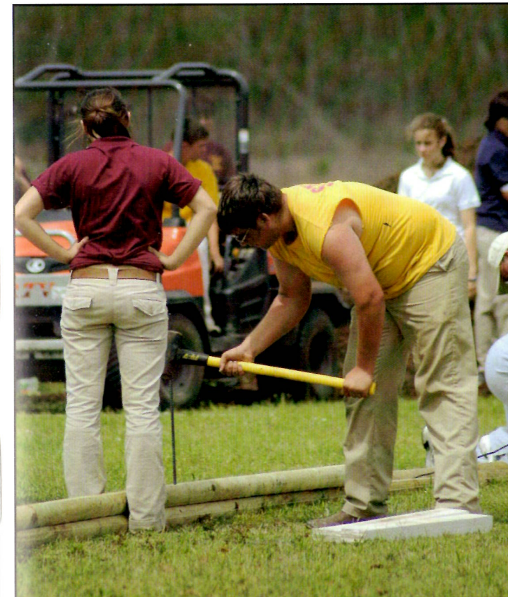
Samantha Williams (10) waits for Clint Guillory (12) to finish hammering rebar into the ground. The agriscience classes helped to build the foundation for a new elementary playground.
