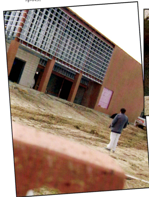
CHAOS ALMOST COMPLETE. When finishing the walls to the gym, everyone was excited to see there is only one more wall to completely close in the gym.
