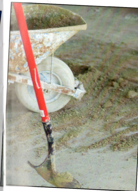
DIGGING DESTRUCTION. After finishing four walls and a roof, there was plenty to be done to the new lobby floor for the new gym.
