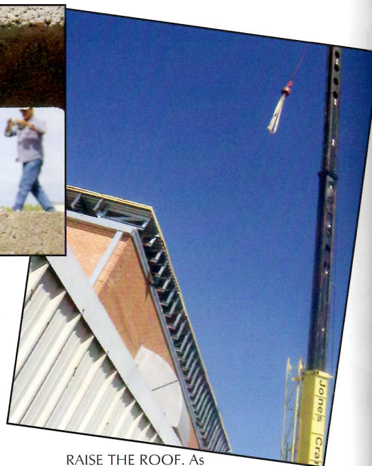
RAISE THE ROOF. As construction workers raise heavy machinery to renovate the new roof, many students became anxious.
